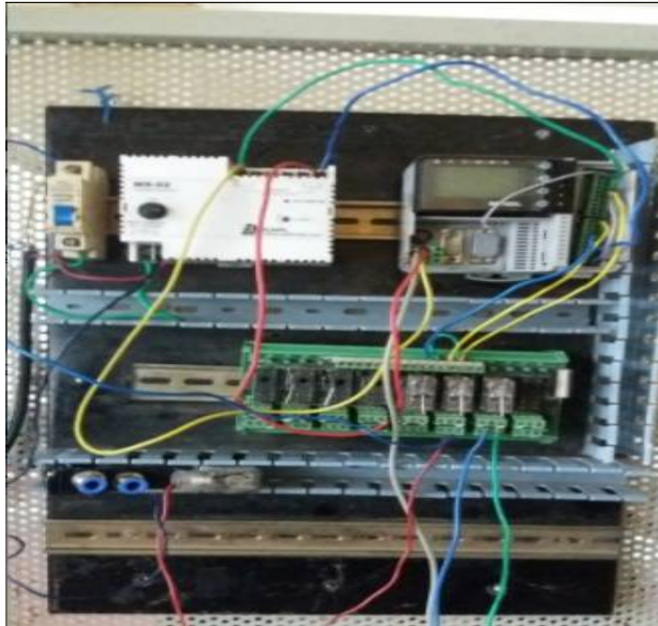
Fig. 5 Hardware Implementation of Project
