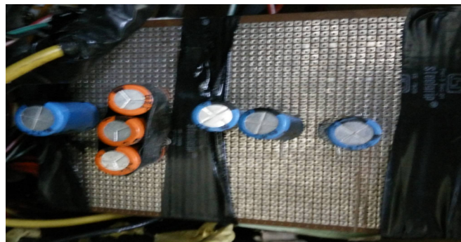
Fig.5(e). Capacitors in regenerative circuit
