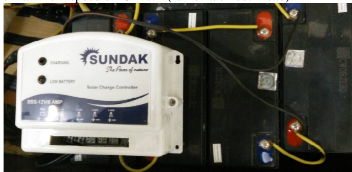
Fig.5(b). PWM charge controller connected to one battery with four batteries connected in series
