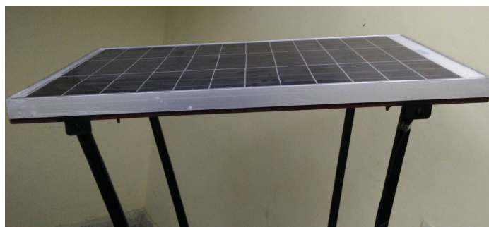
Fig.5(c).One solar panel (12V, 60W) connected to battery
