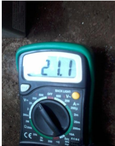
Generator output without load
