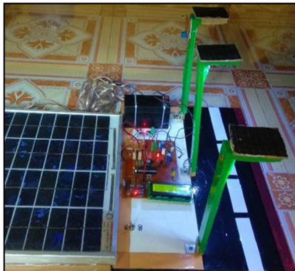
Fig. 4.5 Street Light Is On Condition In night Timing
