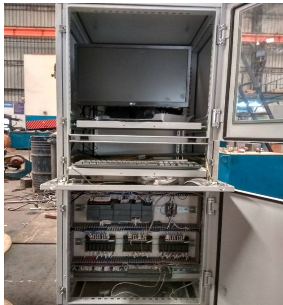
Fig. Control panel picture PLC side
