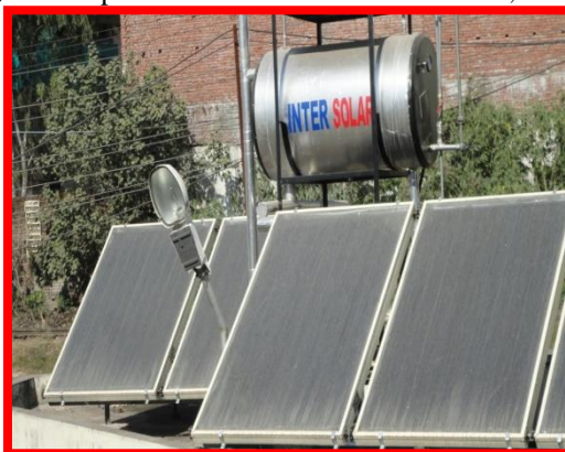
Fig 1: Solar water Heaters
